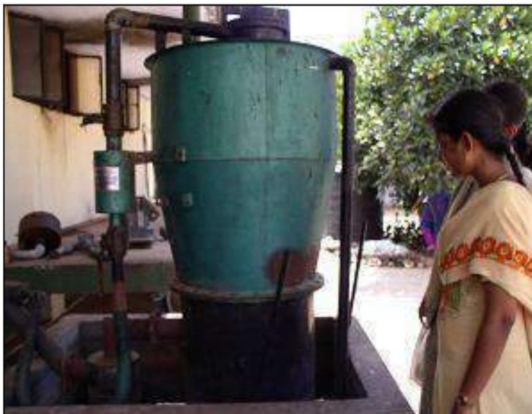
Biomass Thermal Gasifier 20kWe working at our Ladies Hostel]
