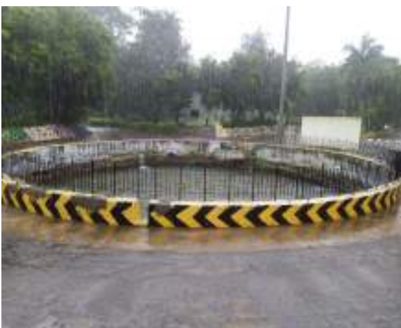
Rain water Harvesting Pond (4250m 3 )
