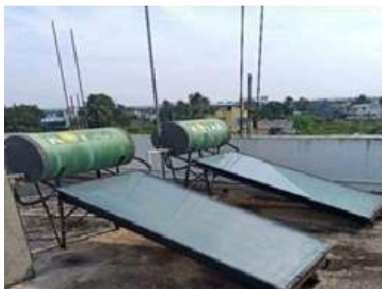
Solar Water Heater
