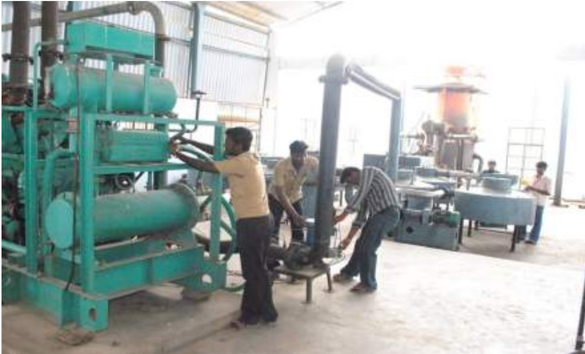
200 kWe bio mass gasifier for power generation (100% producer gas mode) Funded by MNRE, Govt. of India
